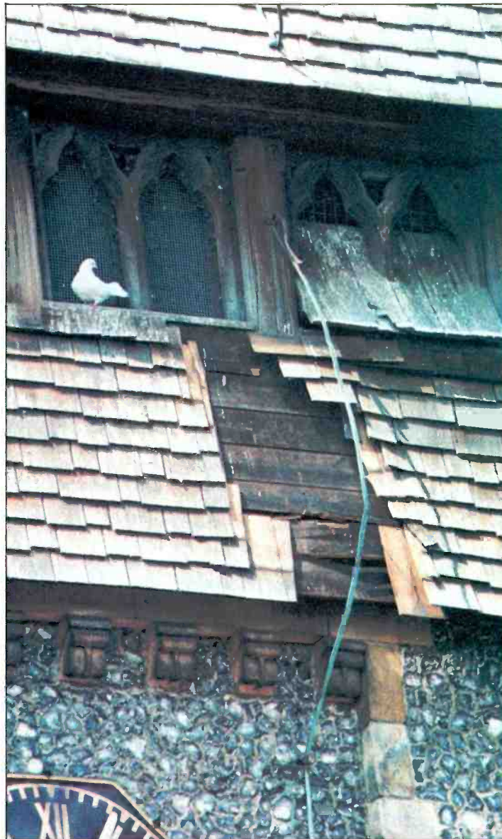
B) Closer view of the damage shown in the heading picture.
